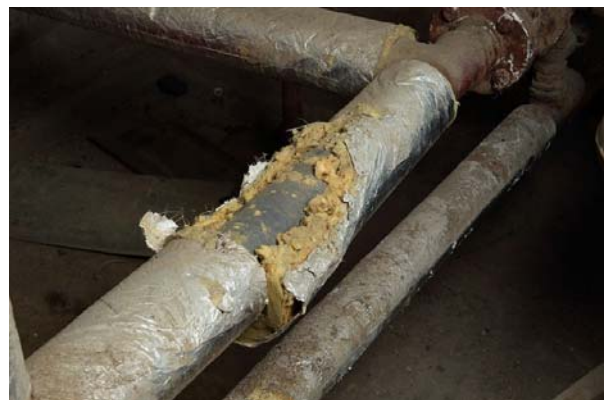
Repair damaged insulation
